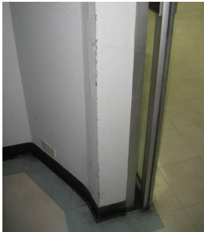
Figure 19: Damage of the Centre's Walls
