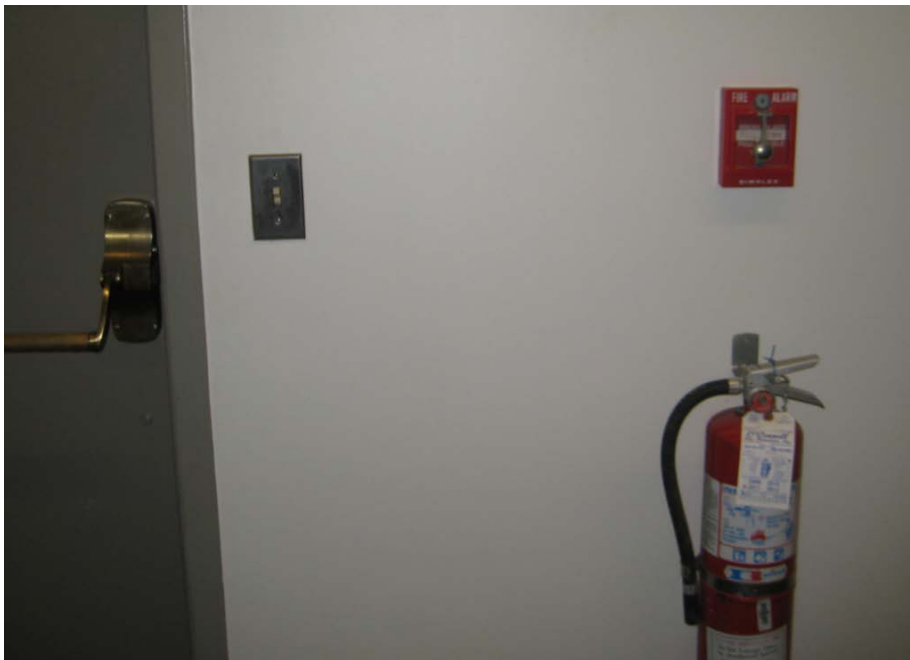
Figure 93: Pull station correct height and distinguishable (items 21 and 22)
