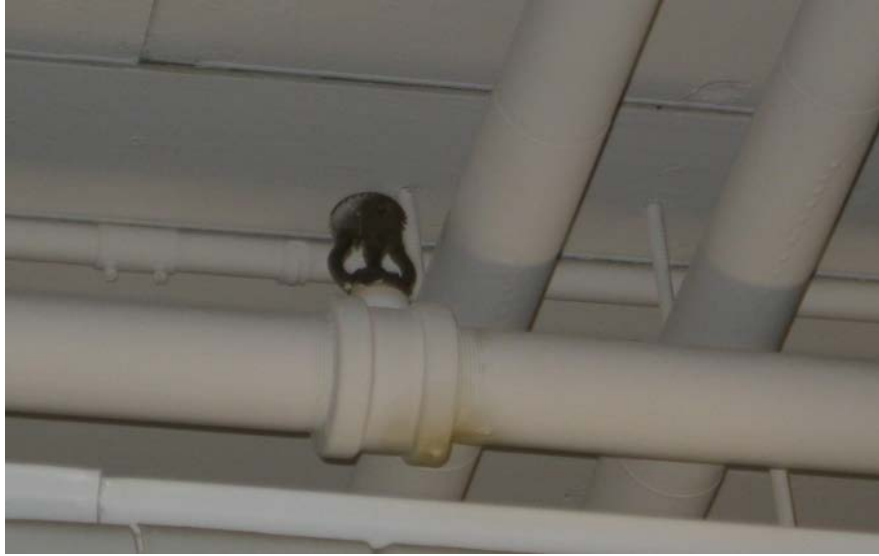
Figure 88: Frame arms parallel to branch line (item 4) Deflector parallel to ceiling (item 7)
