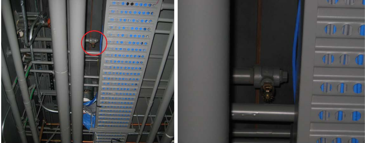
Figure 55: Sprinkler Obstruction in Second Floor Hallway Ceiling
