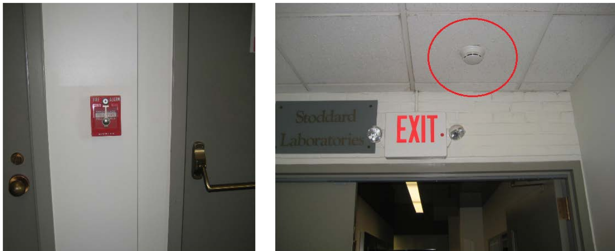
Figure 65: Manual Pull Station and Smoke Detector used in 2011 Roof Renovation Fire
