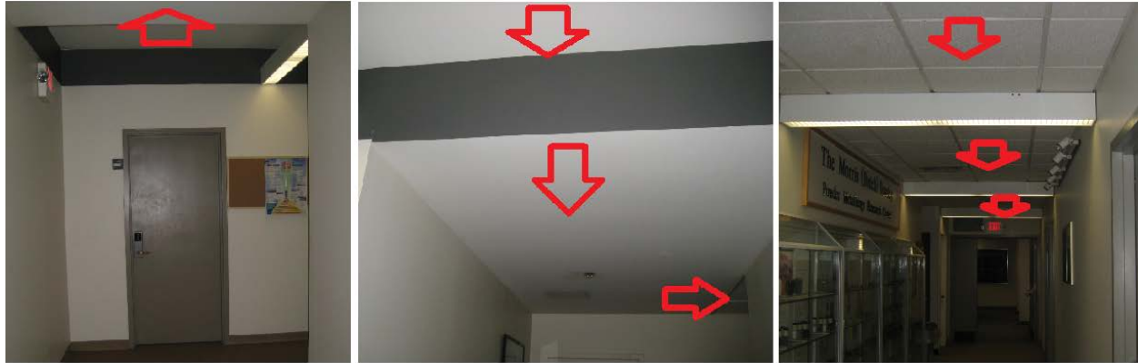
Figure 64: Smoke Pattern of 2011 Roof Renovation Fire
