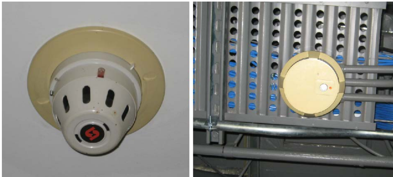
Figure 91: Marked Smoke Detectors (items 18 and 23)
