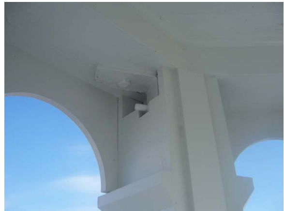
Old Exterior Tower Bracket
