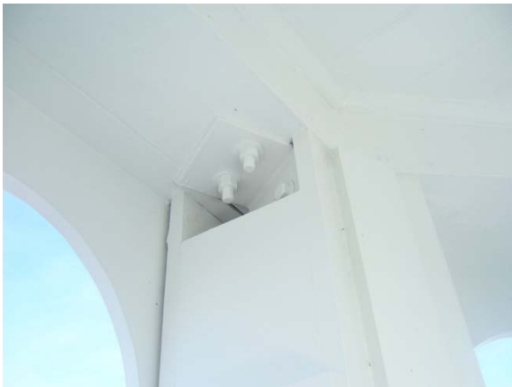
New Exterior Tower Bracket
