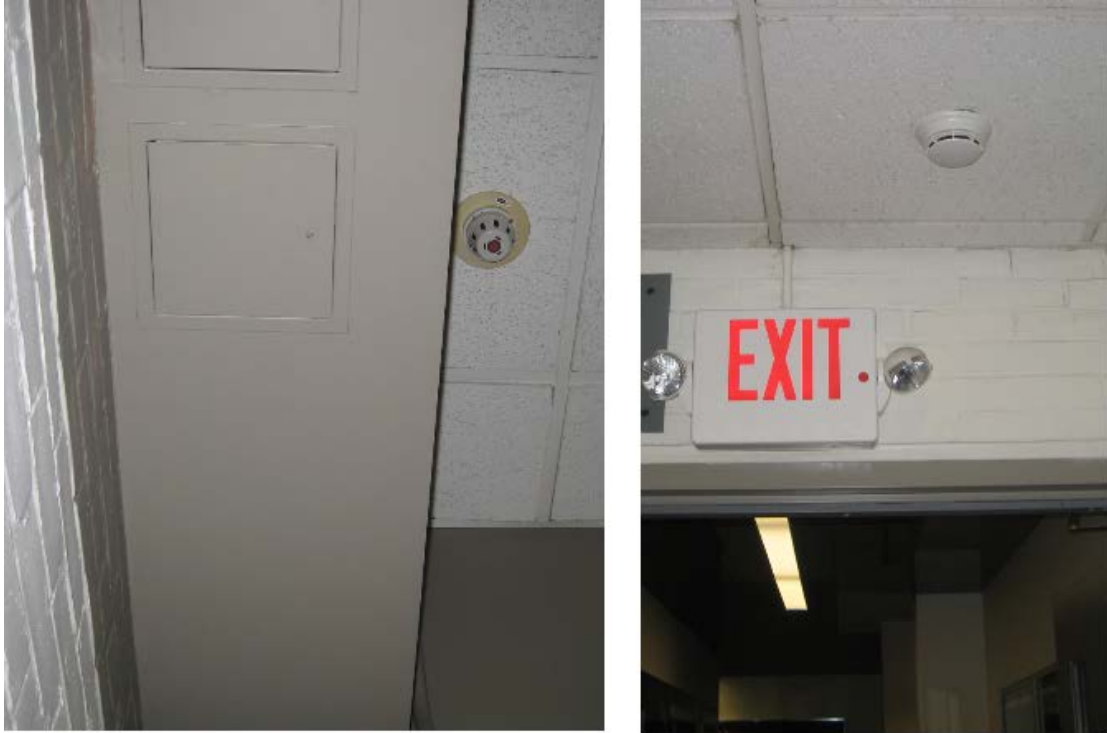
Figure 94: Smoke detectors on either side of fire door (item 24)
