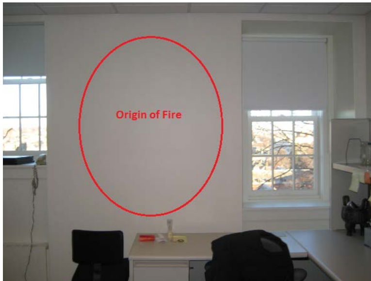
Figure 63: Origin of 2011 Roof Renovation Fire
