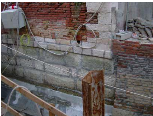
Figure 9: Canal Wall Damage in Venice
