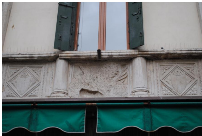
Figure 23: Public art in Venice damaged beyond recognition
