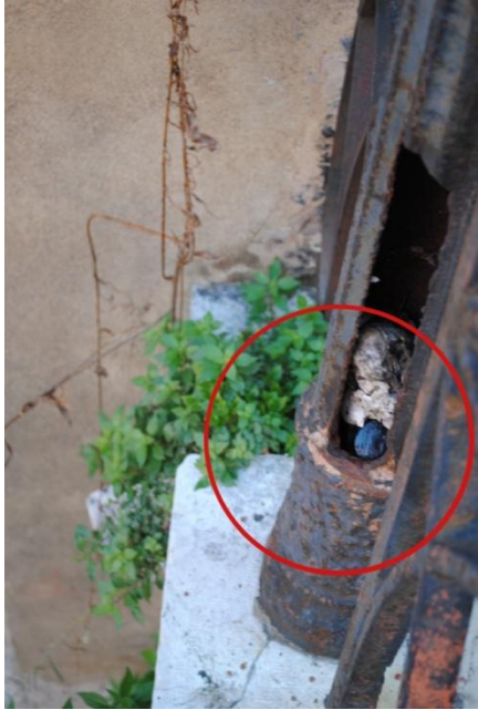
Figure 36: The second container hidden on the Ponte de L'Anzolo
