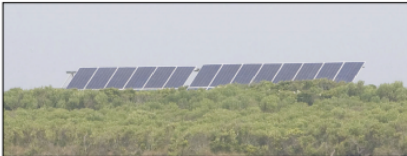
Figure 7: Photovoltaic Ground Array
