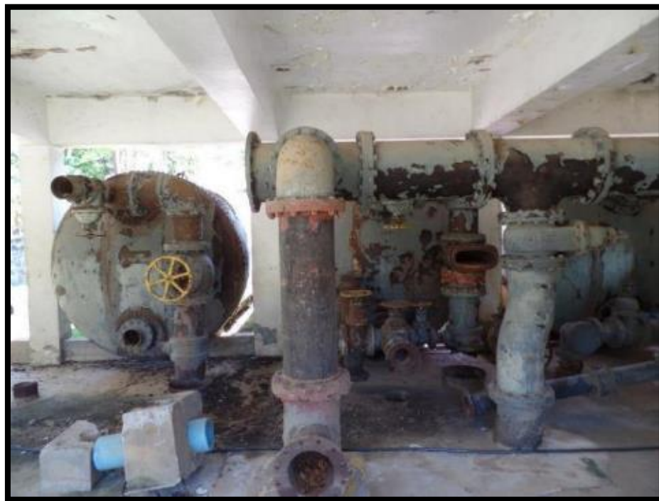
Figure 11. Site of the Antiguo Acueducto. The current condition of the mechanical water filtration system.
