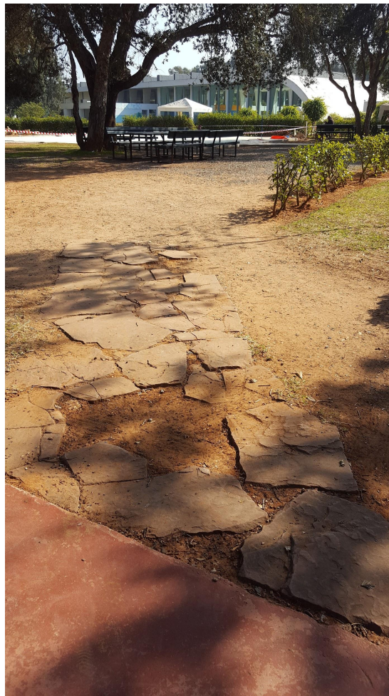
Figure 4.16. Gravel pathway that is not accessible for everyone.
