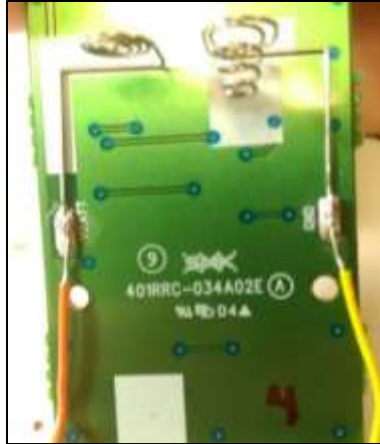
Figure 20: Wires Soldered into Power Supply
