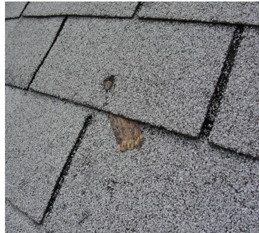
Figure 3: Roof Damage on an Asphalt Shingle
