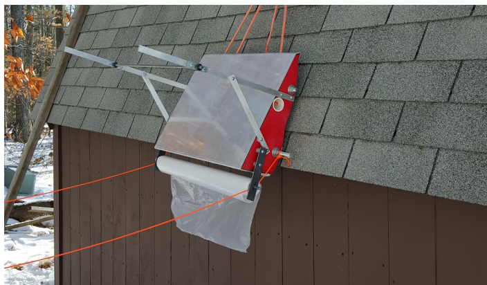
Figure 49: Wedge on the Roof
