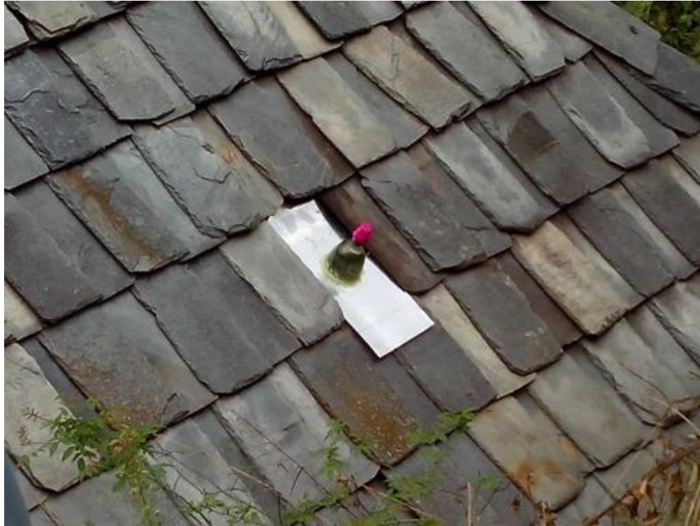
Figure 32: Solar bottle bulb implemented on a roof. The nail is not visible because the upper two slates are covering it. (Photo credit: Siddhant Mohan, 2013)
