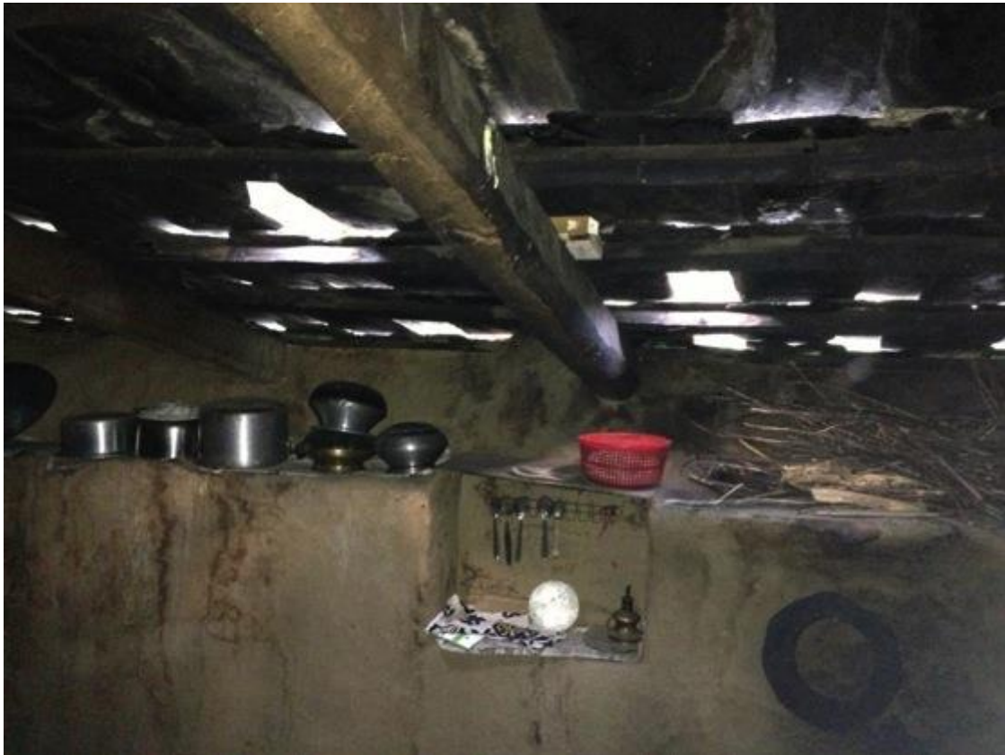
Figure 30: The house with no ceiling - slate structure (Photo credit: Mert Can Erad, 2013)
