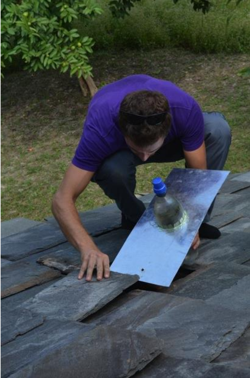
(Photo of team member Mert Erad fitting the solar bottle bulb into the roof)
