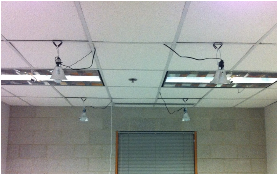
Figure : Overhead light setup
