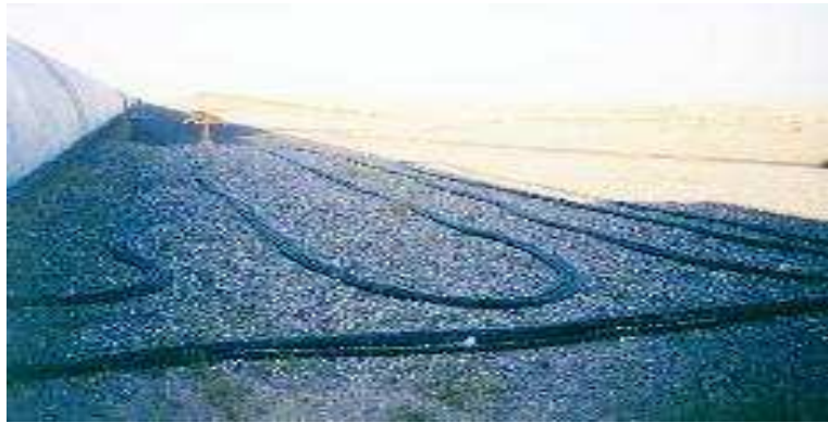
Figure 14: Copper Cables for Heating Tube
