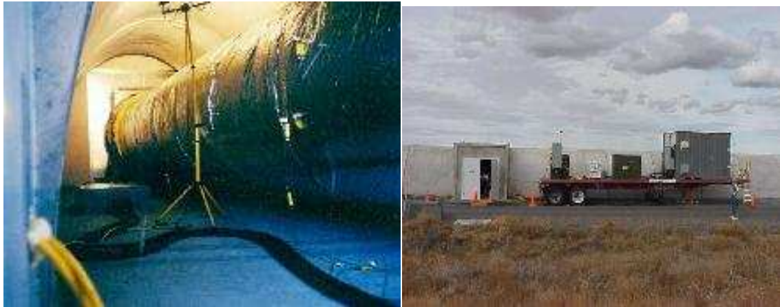
Figure 13: Left - Fiberglass Insulated Tube, Right - Power Supply for Tube Heating
