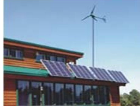
Figure 1 – Small Wind Turbine
