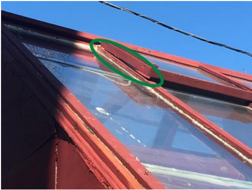
FIGURE 3 LEAK IN THE GREENHOUSE ROOF
