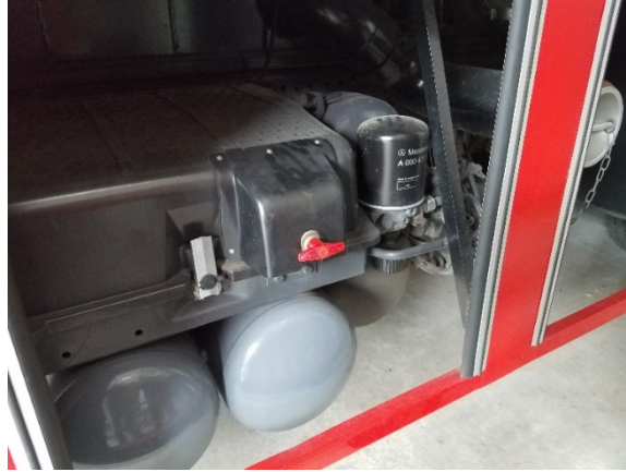
Figure 20 Auxiliary Power Unit
