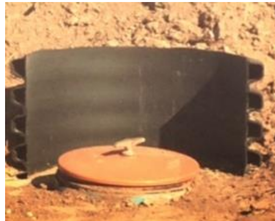
Figure 15: Bubbler valve used in Santa Ana
