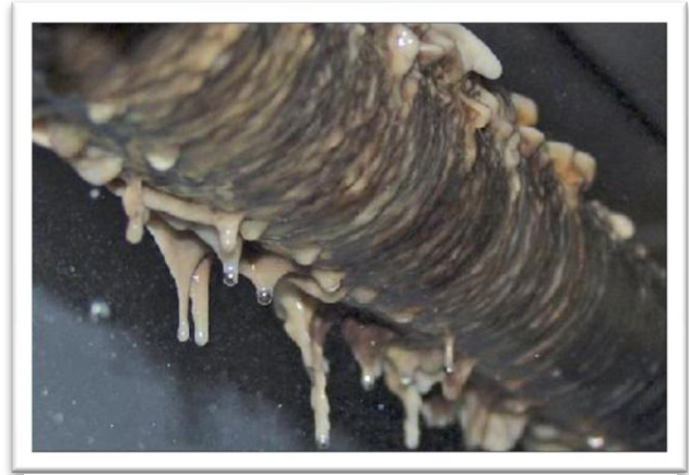
Figure 2-6 – Chemical biofouling of a pipe in a factory [3]
