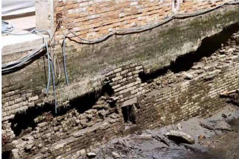
Figure 12: A damaged canal wall 33
