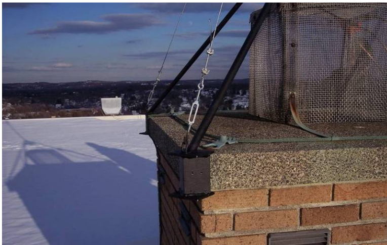
Figure 33: Guy Wire Turnbuckle Connection
