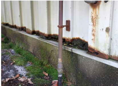
Figure 27: Rusting building shell
