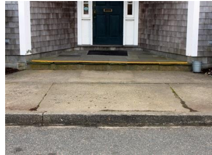
Figure 29: Non-ADA compliant entrance
