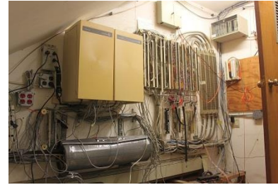
Figure 34: Messy IT room
