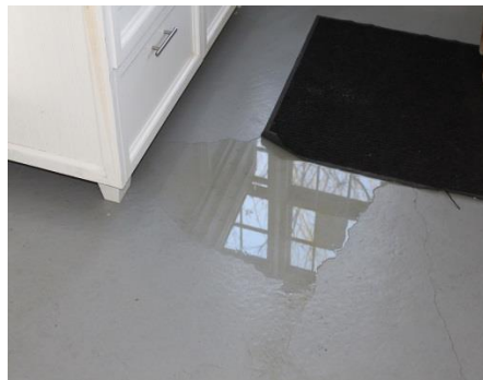
Figure 60: First floor flooding
