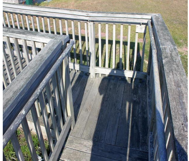
Figure 20: Tight ramp at DPW Administrative Building
