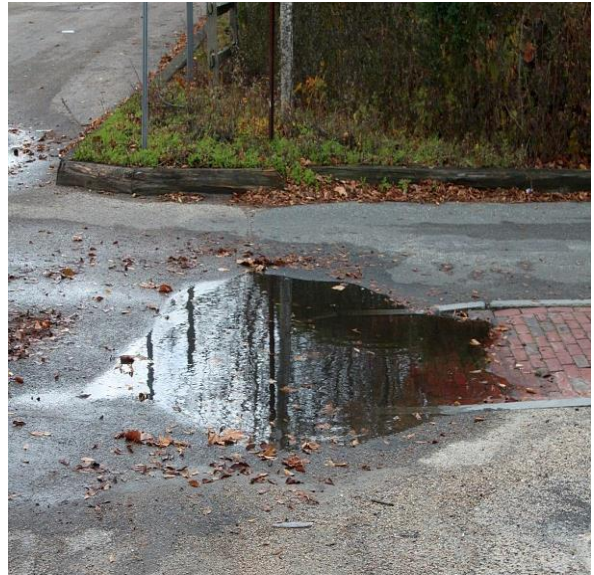
Figure 18: Poor drainage at the Finance Building
