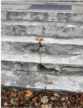
Figure 82: Deteriorating concrete staircase
