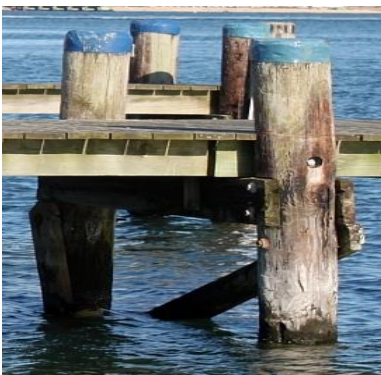
Figure 44: Broken bracing/rotting pylon
