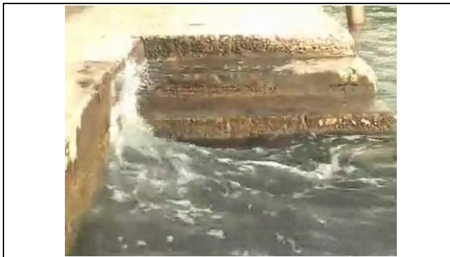
Figure 26 - Venetian steps and walkway being eroded by saltwater of canals lapping against them
