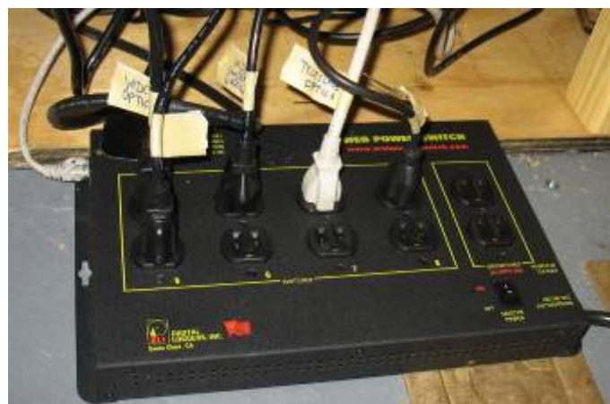
Figure 10: Web Power Switch Installed On-Site
