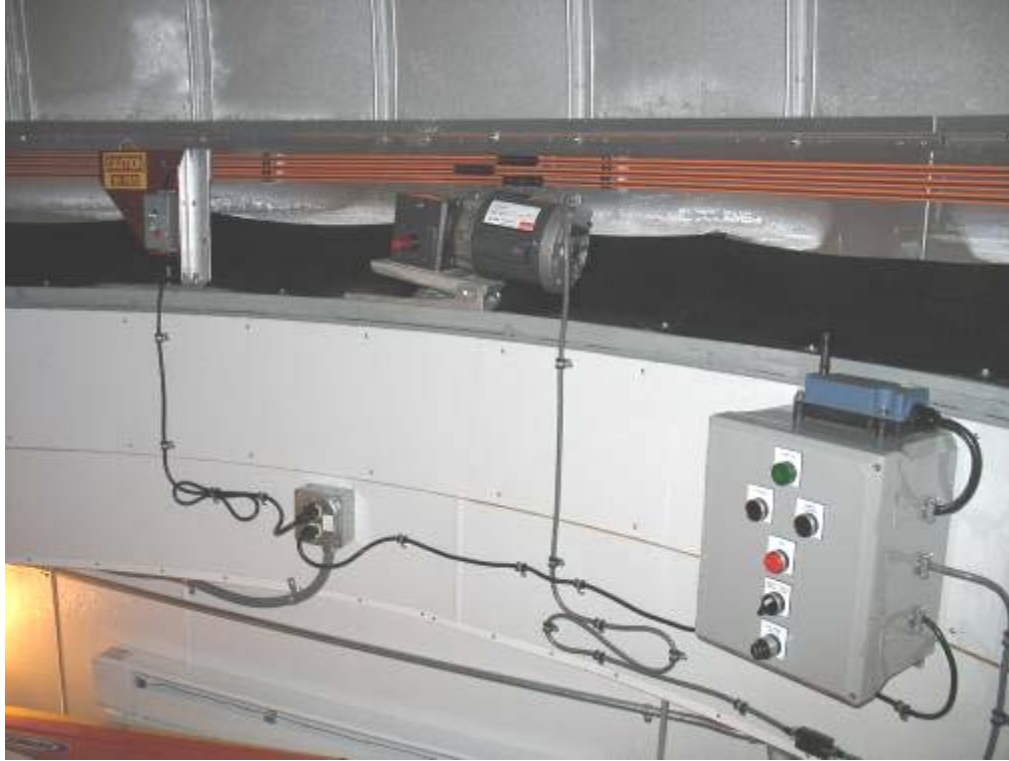
Figure 13: Dome rotation controller and motor are mounted to the building and are stationary
