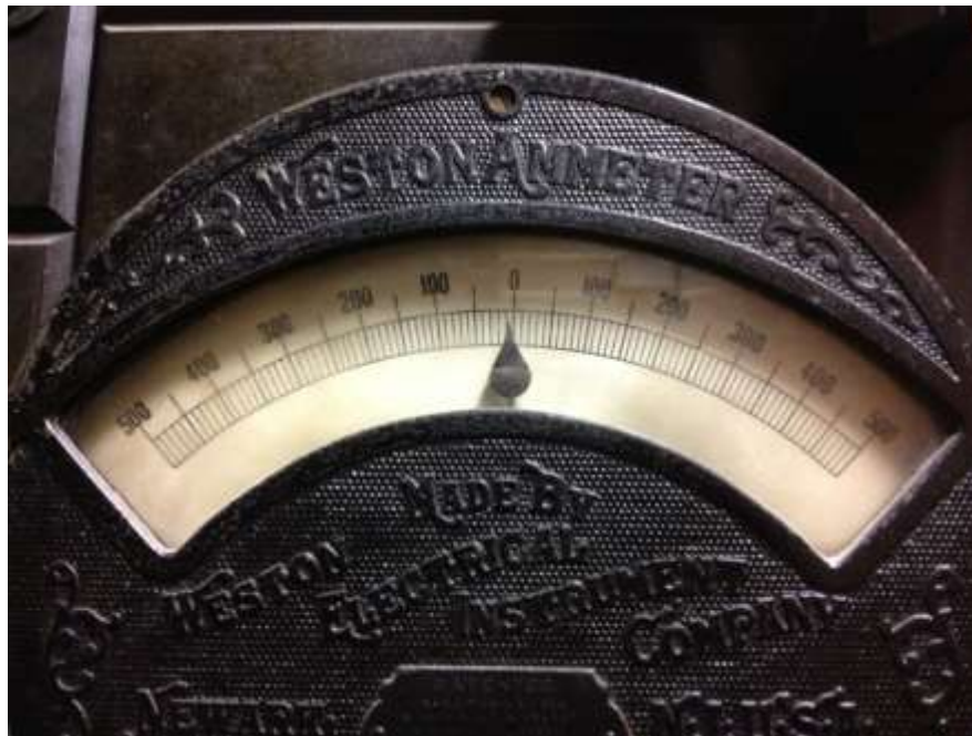
Figure 31: Ammeter portion of electrical control panel
