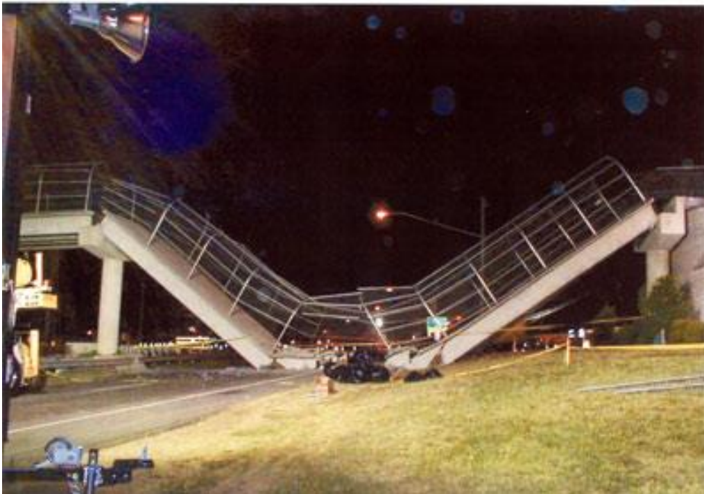
Figure 10: Simply-Supported Pedestrian Bridge Failure, Lowes' Motor Speedway, North Carolina
