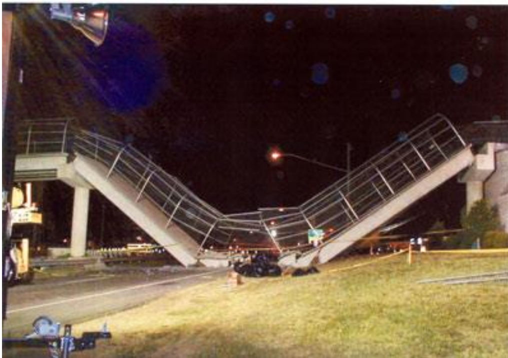
Figure 37: Simply-Supported Pedestrian Bridge Failure
