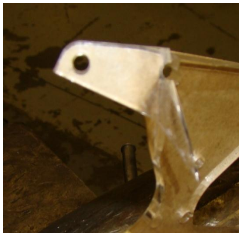
Figure 62: Crack in Body Plate
