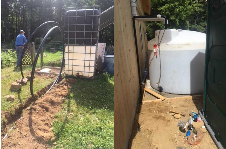
Figures 21 & 22: Construction Day 3: Piping Leading to Overflow and Irrigation Connection (left) and Profile of Barrel Where White Is Collection Pipe and Black Is Delivery Pipe (right) Image Source: Virginia Adams
