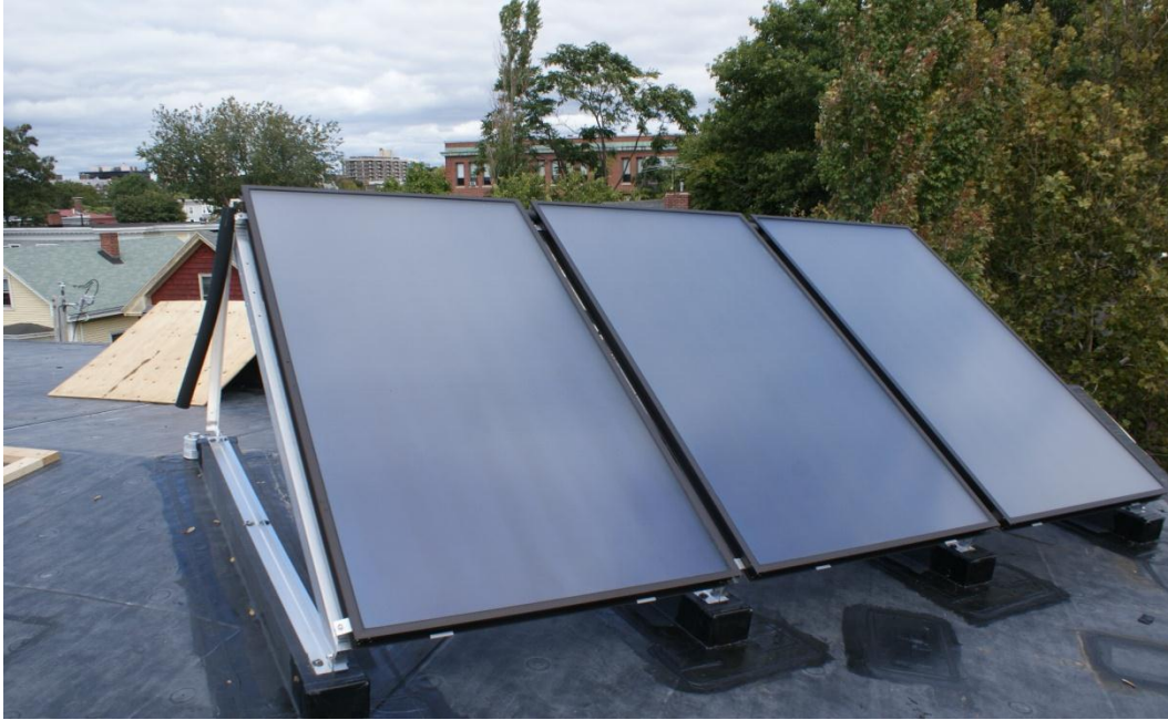
Figure 5. Three Schuco Slim V Collectors on a Tilt Rack, Cambridge, MA
