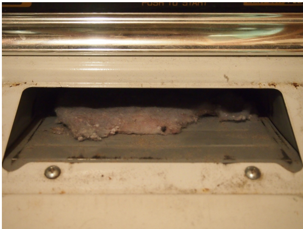
Figure 3: Result of Uncleared Lint Screen: Clogged Lint Area
