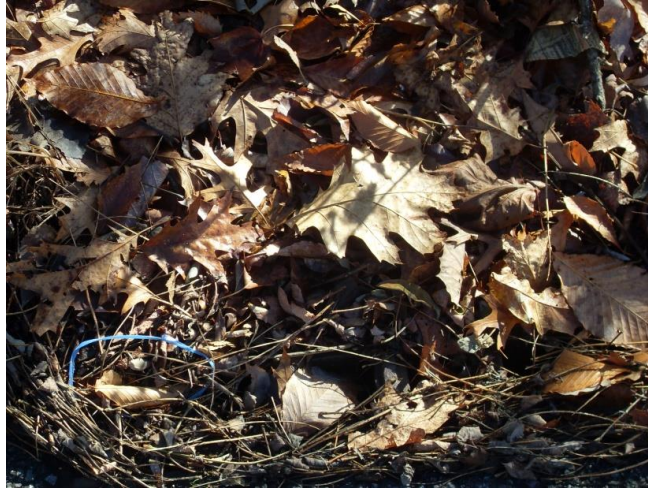
Figure 8: A catch basin in Leicester completely hidden by leaves (November 18, 2013)
