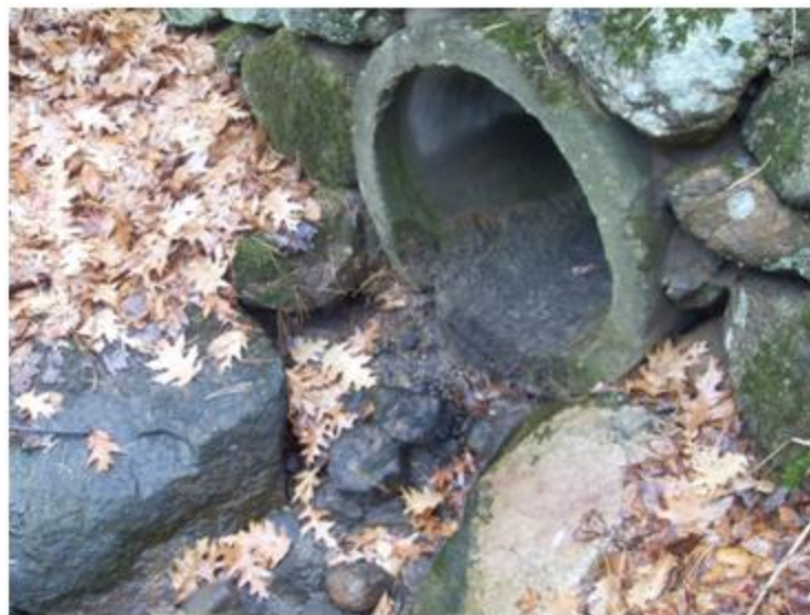
Figure 12: Outfall in Upton with abrasion due to excessive sediment (Nov. 22, 2013)
