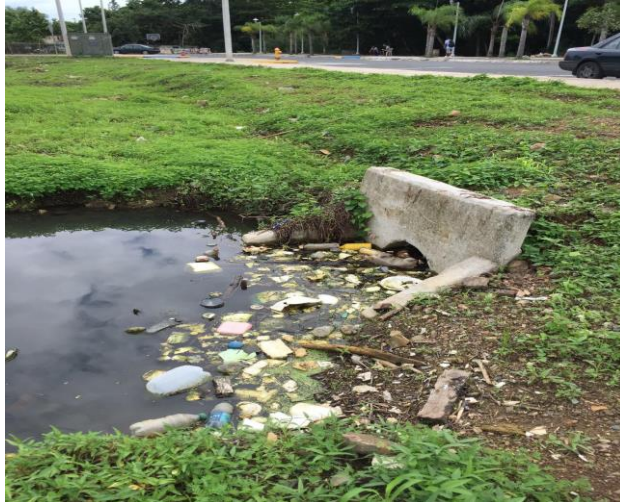
Figure 4: Clogged Drain in Cantera
