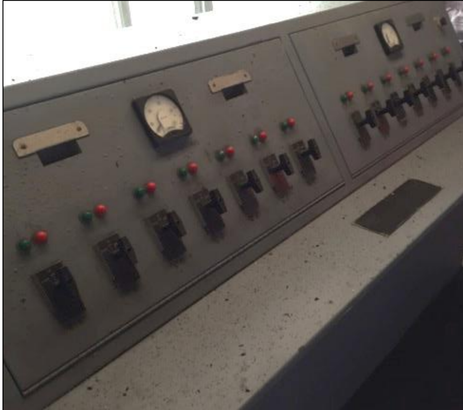
Figure 76: Control desk where the spillway gates are opened and closed
