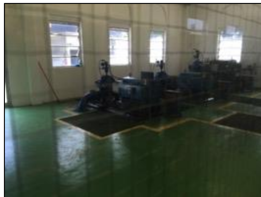
Figure 49: Water Pumping Station
