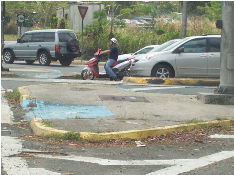
Figure 64: 199 & 876 Intersection Pedestrian Islands
