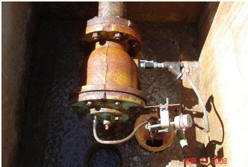
Figure 15: An actual automated bulb controlled valve found on a PRASA tank.
