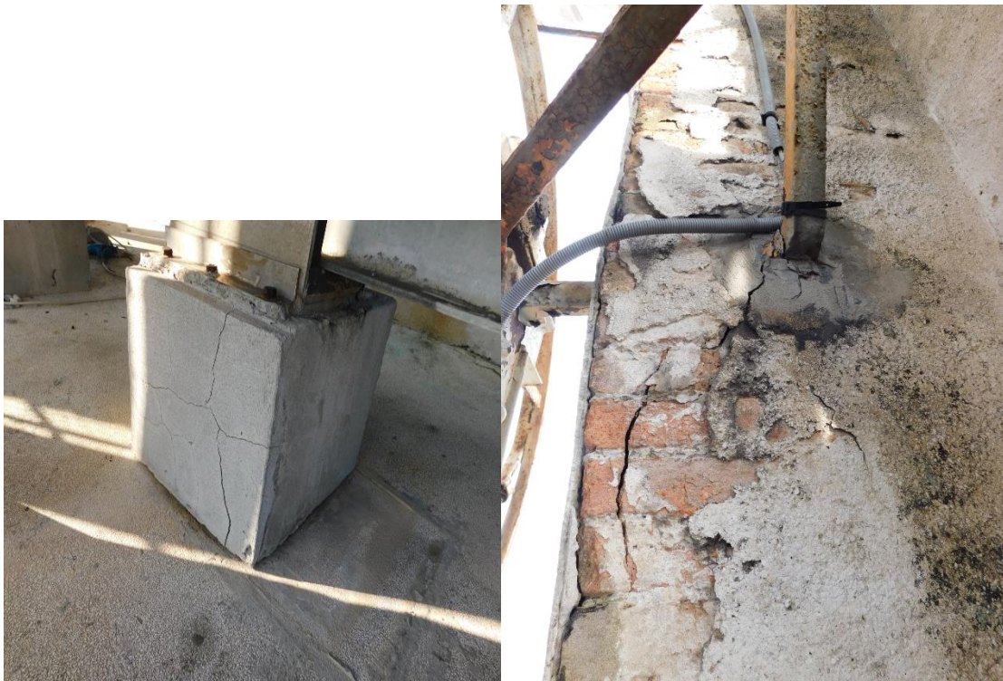
Figure 62 - Cracks from the bell frame in San Giacomo dell’Orio (left) and Gesuati (right)
