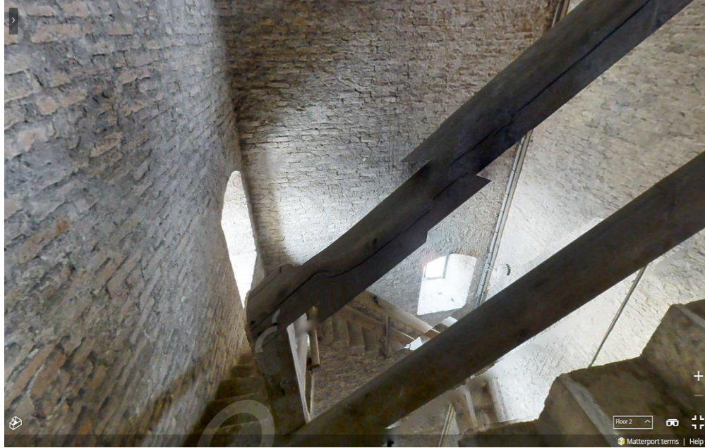
Figure 77 - MatterPort stitching error. The railing in this scan is noticeably misaligned.
