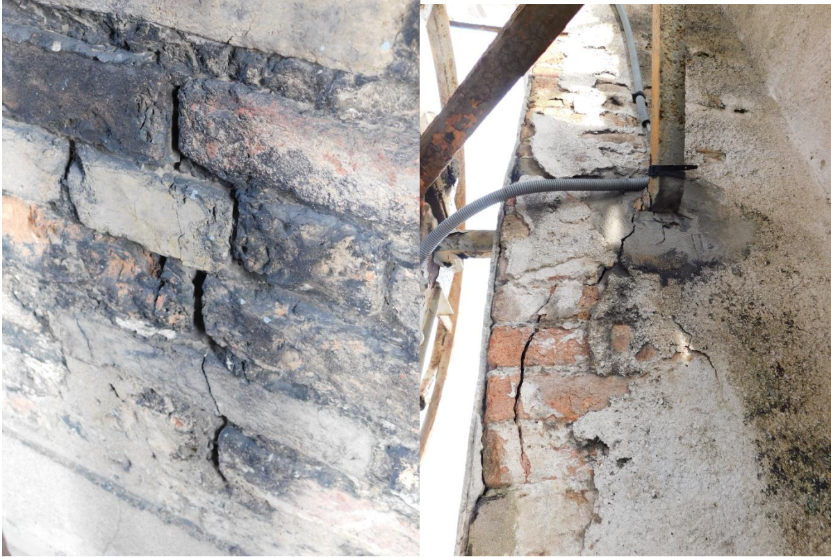
Figure 23 - Examples of an insignificant (left) vs. a significant (right) crack
