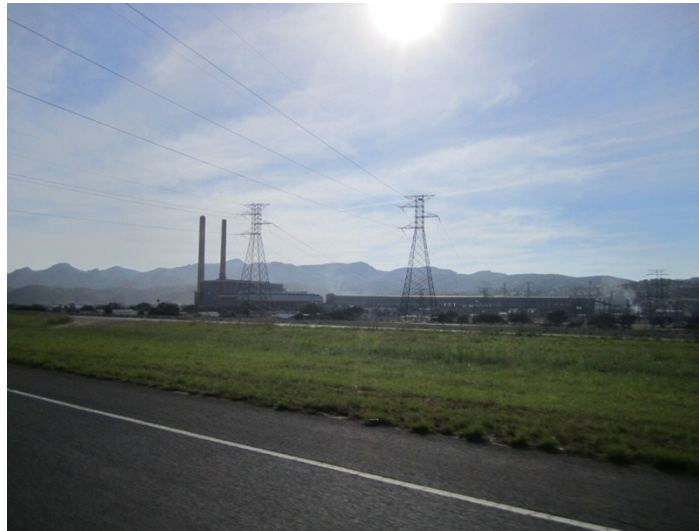
Figure 13: Coal power plant outside of Windhoek
