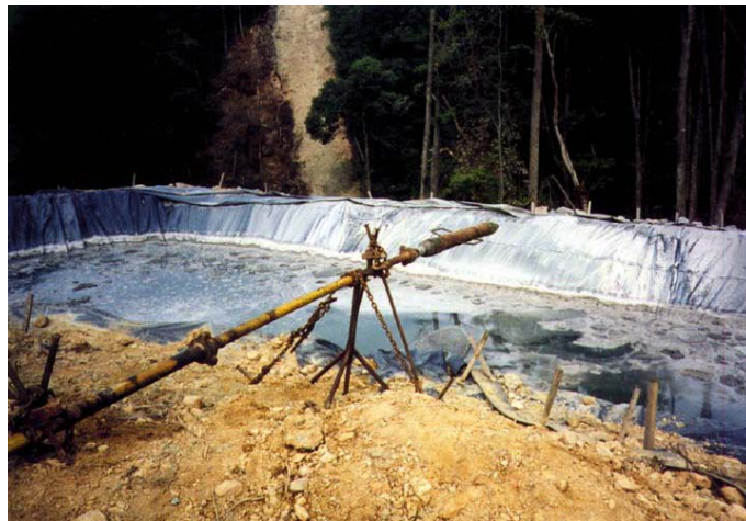
Figure 3.9: Fluid that is extracted from the well during drilling or production is stored in a lined trench until treatment. This also shows the clearing of land that must occur to account for the trenches. lxxxiii
