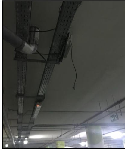
Figure 13: Electric wires hanging in Morocco Mall underground parking garage
