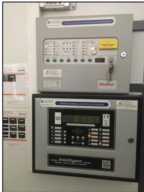
Figure 28: Fire panel in the Mondi administration office
