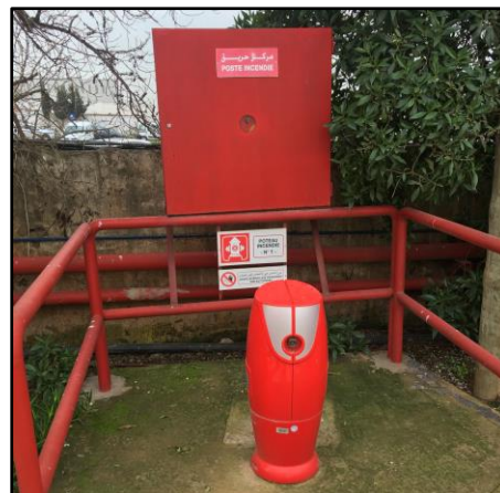
Figure 32: Water hydrant and attachable hose located next to the outdoor storage area
