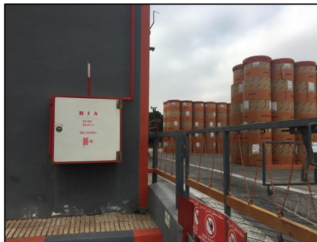
Figure 30: A fire hose next to the Mondi outdoor storage area
