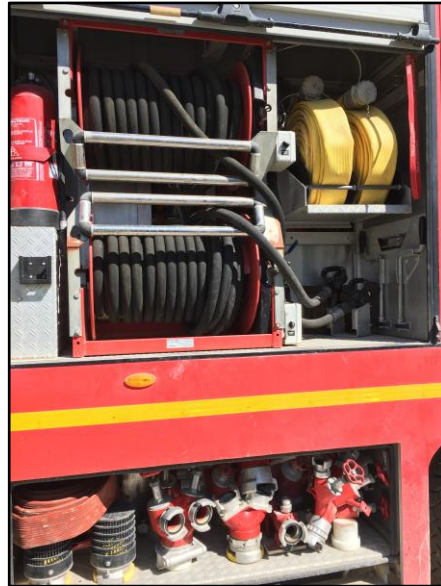
Figure 46: Hoses in OCP fire truck used for large scale fires and extra valve replacements
