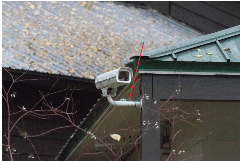
Figure 19: Apgar Village webcam with ethernet cable
