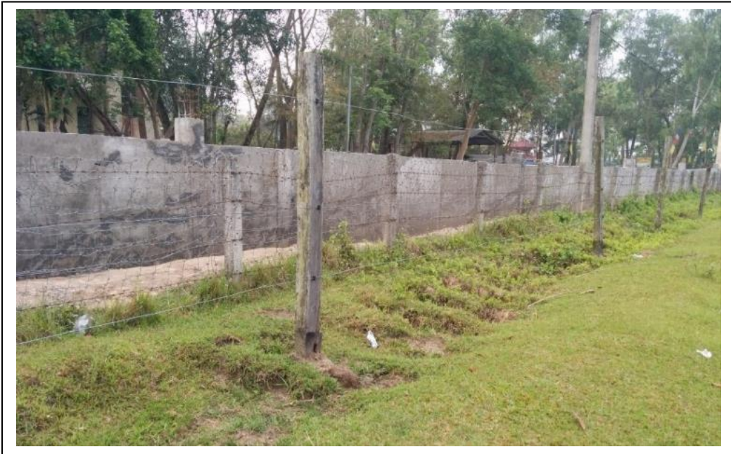
Figure 5.12- Ongoing constructio of concrete wall in buffer zone and aournd Bagmara CF (Photo by Yogesh Dongol)
