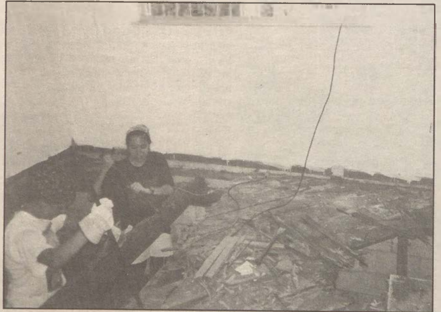
Jen Vincola and Ellie Cooper use crow bars to destroy a termite-eaten floor and later replace it with a new one.
