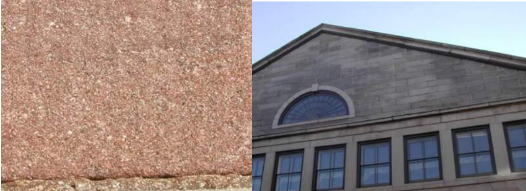
Figure 33: Local red sandstone of Portland (source by Department of Agriculture, Conservation & Forestry)
