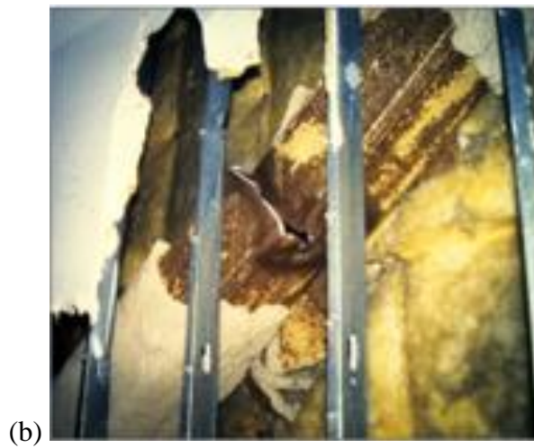
Figure 2-2. Damages in building structures during the 1994 Northridge Earthquake: (a) the 4-story steel framed HP building (Hall et al., 1995); (b) damaged brace was revealed after the dry wall has been removed (Sabelli, 2013)
