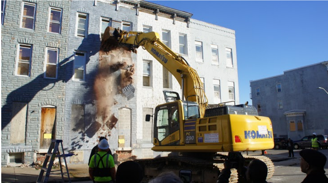
Figure 6. Project C.O.R.E. demolition began in January 2016 in Sandtown-Winchester. Digital Image. Maryland Department of Housing and Community Development. January 5, 2016.
