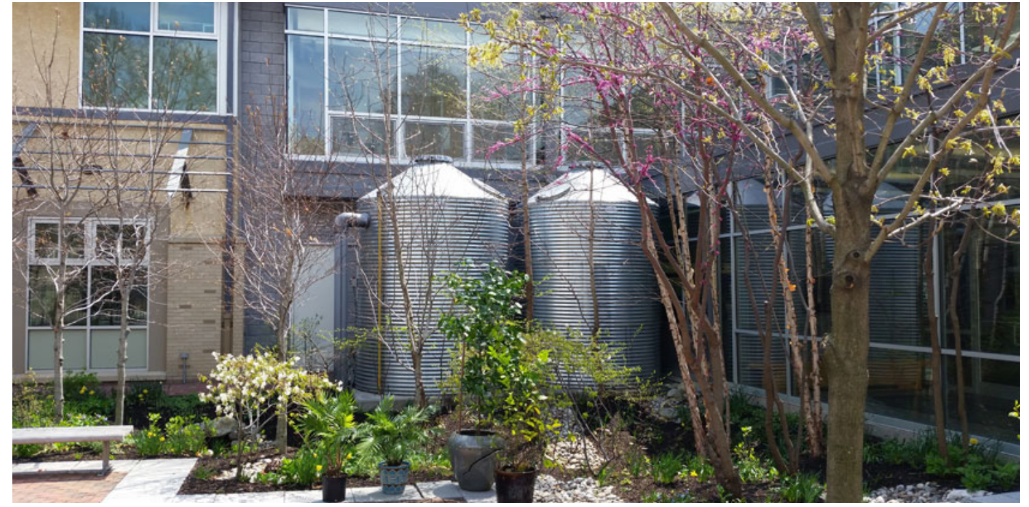
Figure 4. Cisterns in Use Surface cisterns located outside of a building in Philadelphia. (www.pwdplanreview.org)
