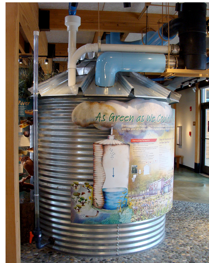
Figure 8. Rain Water Harvest Cistern (www.aiachicago.org) Educational and environmental feature within the site that holds 1,500 gallons of rain water.
