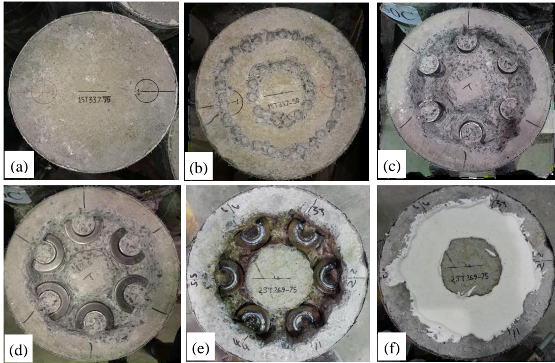
Figure 6.12: Remedial measure for the slip of steel tubes: (a) specimen before repairing; (b) drilling of concrete cover; (c) specimen after removing concrete cover above tubes; (d) washers fitted on tubes; (e) welding of washers; (f) plaster infill.
