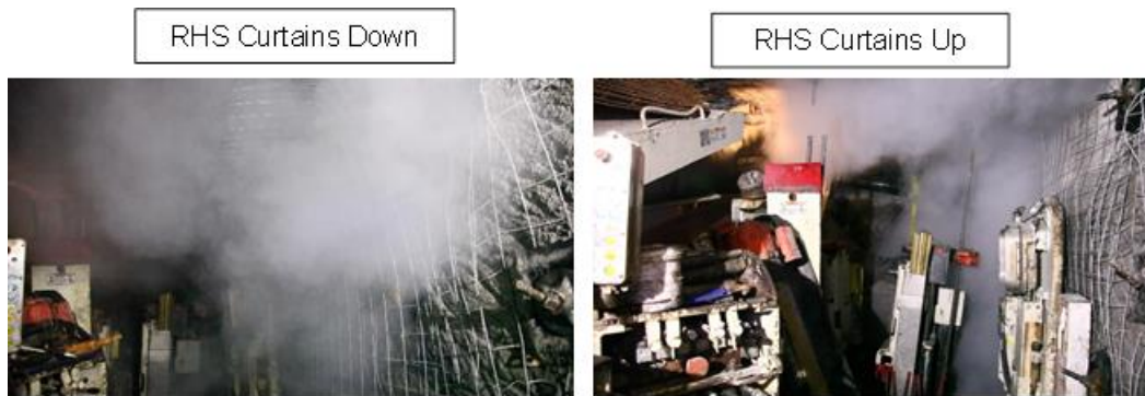
Figure 5: RHS curtains down and curtains up dust migration
