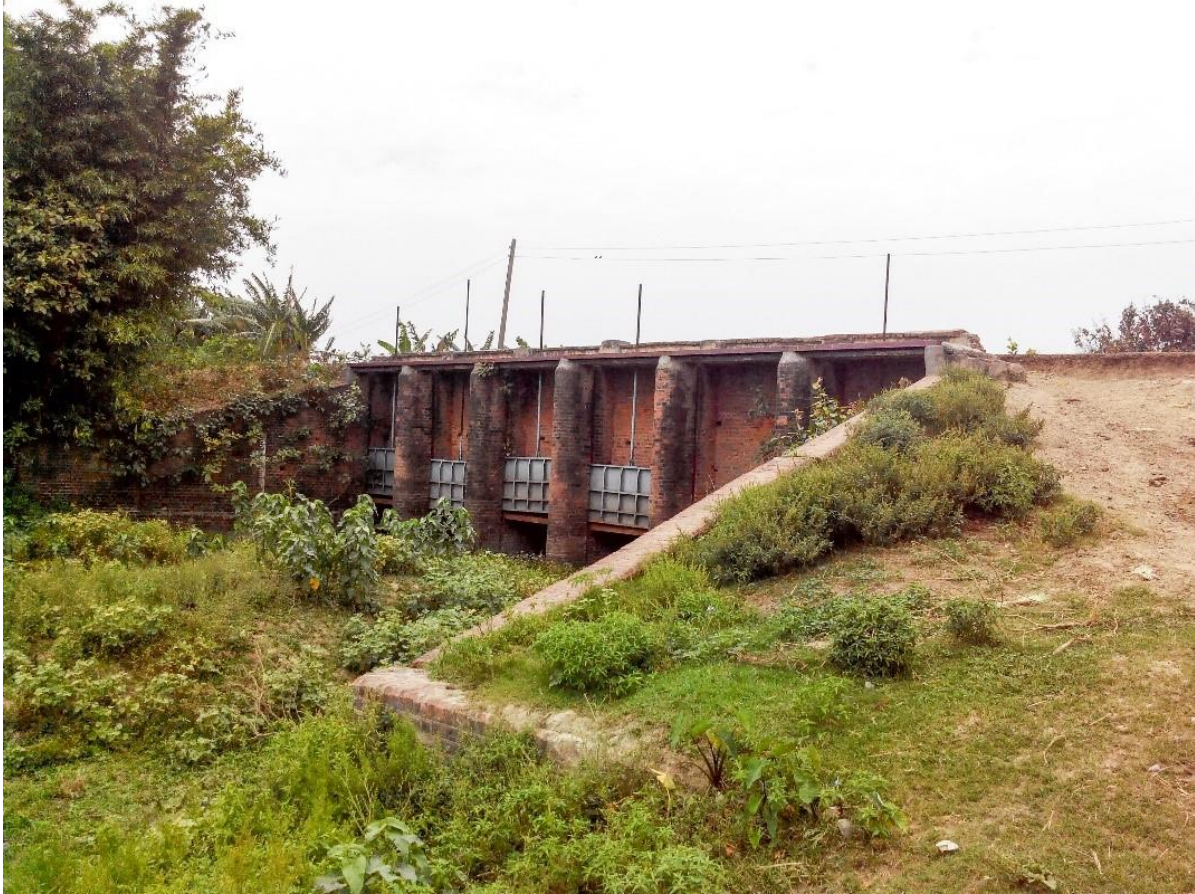
Photograph 6.10: A non-functional sluice gate along the western embankment in Hanumannagar
