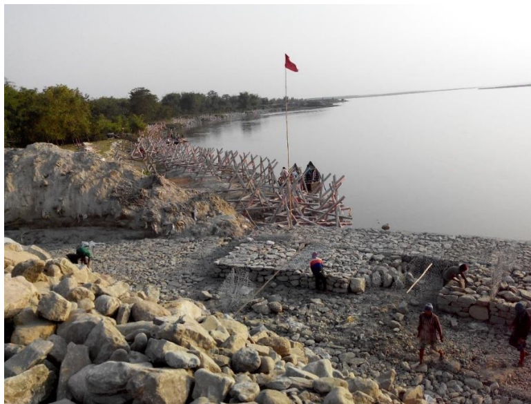
Photograph 6.11: Construction of Porcupines and a spur along the eastern bank of the Koshi River in Prakashpur
