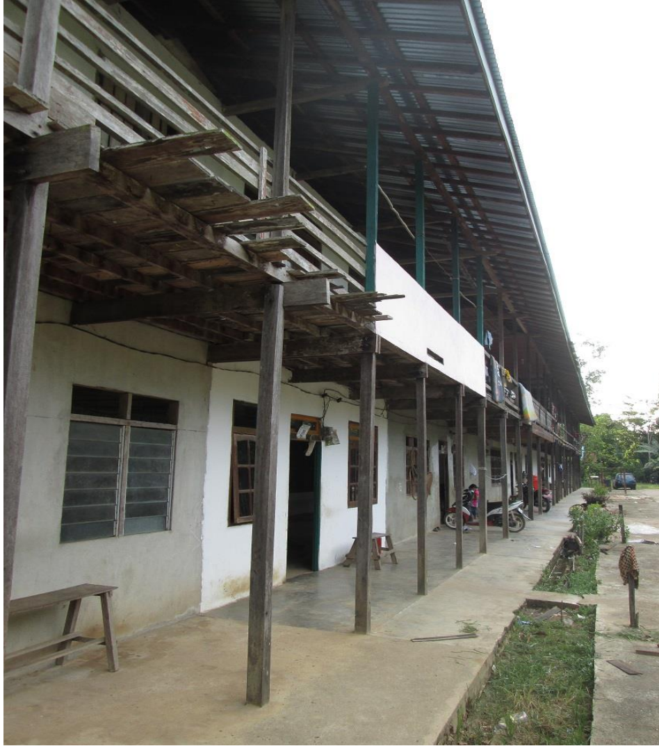
NB: Some of the longhouse walls have been renovated with cement to reduce any future risk of fires
