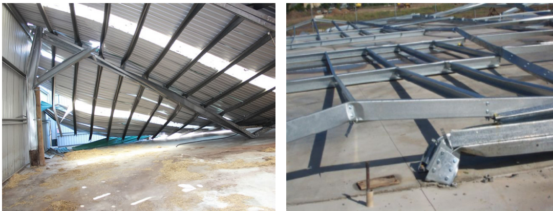
Figure 1.3: Failures of cold-formed steel structures
