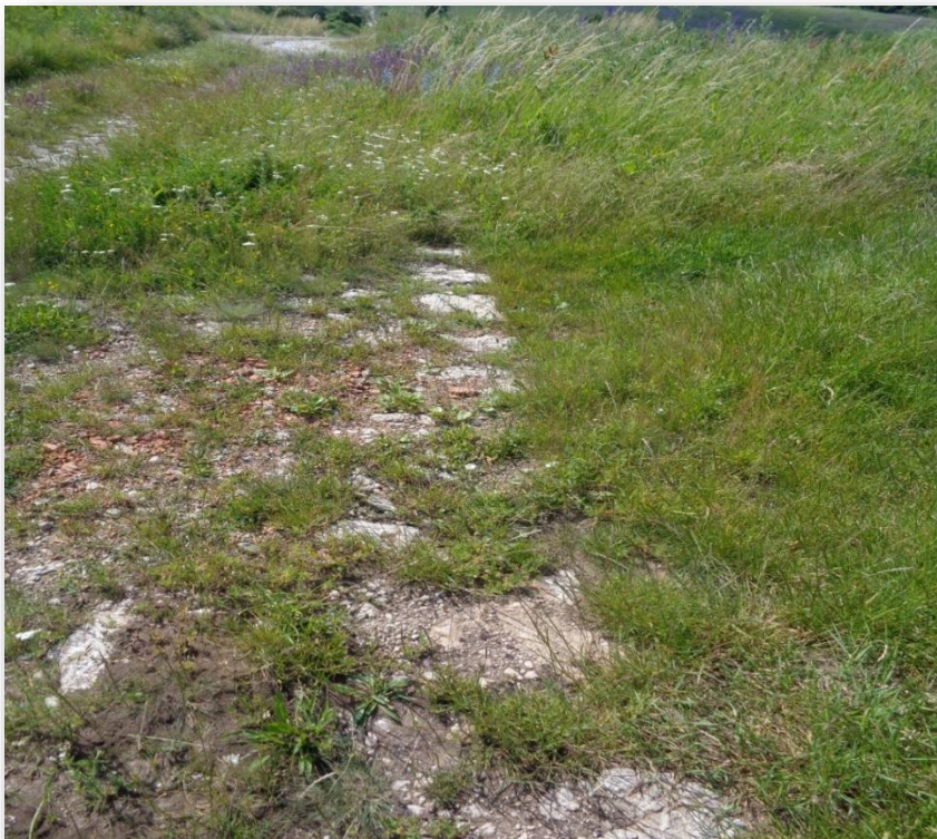
Figure 33: Exposed pavement of the road as it nears Dragoman.
