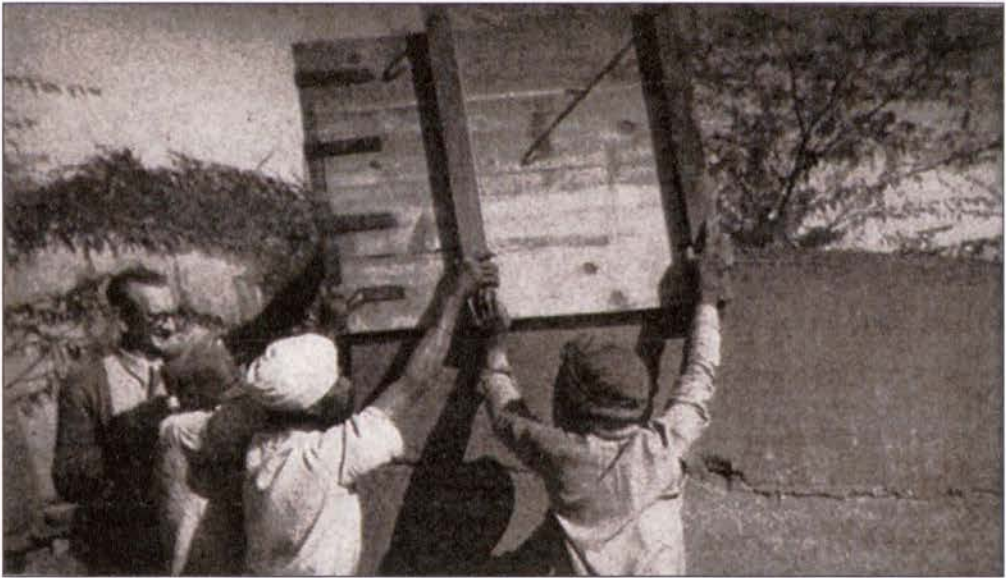
Figure 4.32 Architect Middleton helping the construction workers to remove the mould he designed for rammed-earth wall construction. 139
